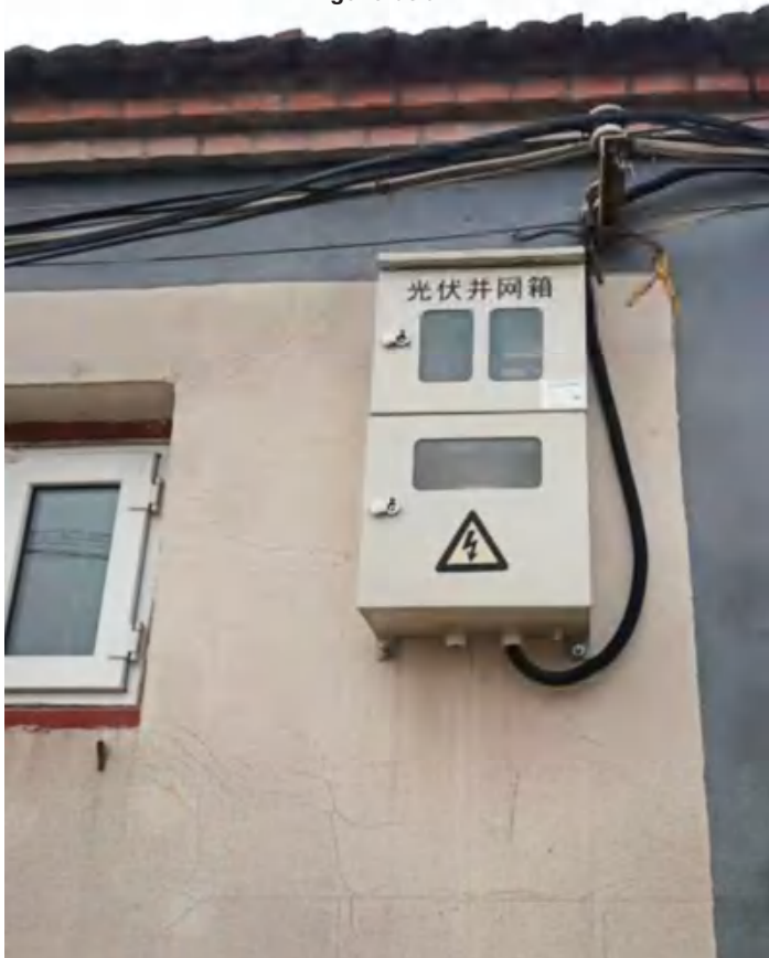
Solar photovoltaic grid connection box
